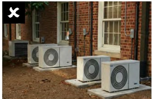
Unshielded ground-level equipment
