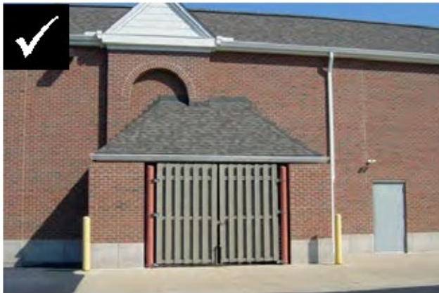
Screened ground-level equipment
