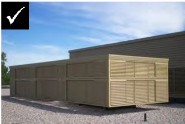
Screened roof-top equipment
